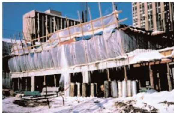
Fig. 1. When suitable preparations to build enclosures and insulate equipment have been made, cold weather is no obstacle to concrete construction.
