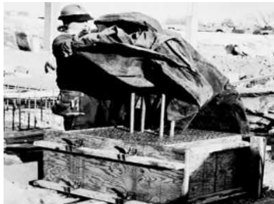
Fig.8. Concrete footing pedestal being covered with a tarpaulin to retain the heat of hydration. Thermometer readings of the concrete's temperature will tell whether the covering is adequate. The heat liberated during hydration will offset to a considerable degree the loss of heat during placing, finishing, and early curing operations. As the heat of hydration slows down, the need to cover the concrete becomes more important.
