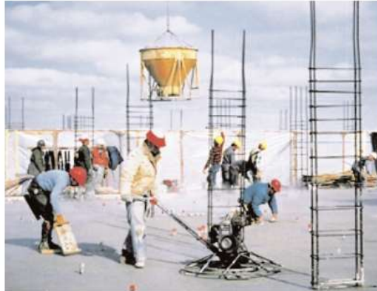
Fig. 9. Finishing this concrete flatwork can proceed because a windbreak has been provided, there is adequate heat under the slab, and the concrete has low slump.
